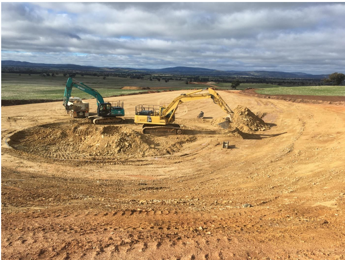
Figure 2 View from BU12 during foundation excavation, in the background BU13 (LHS) and BU14 (RHS).
